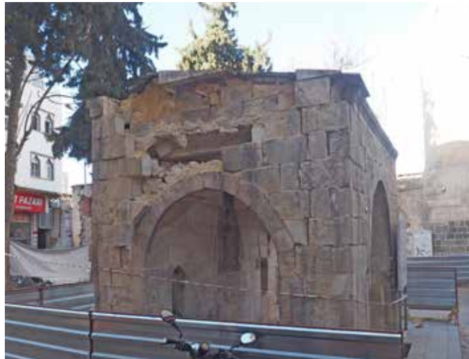
View 2.13 Salih Ağa Fountain after the earthquake
