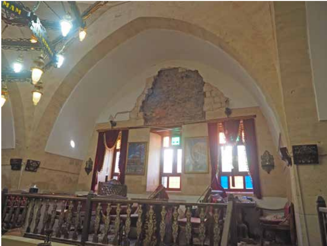
View 2.11 Eski Hamam after the earthquake
