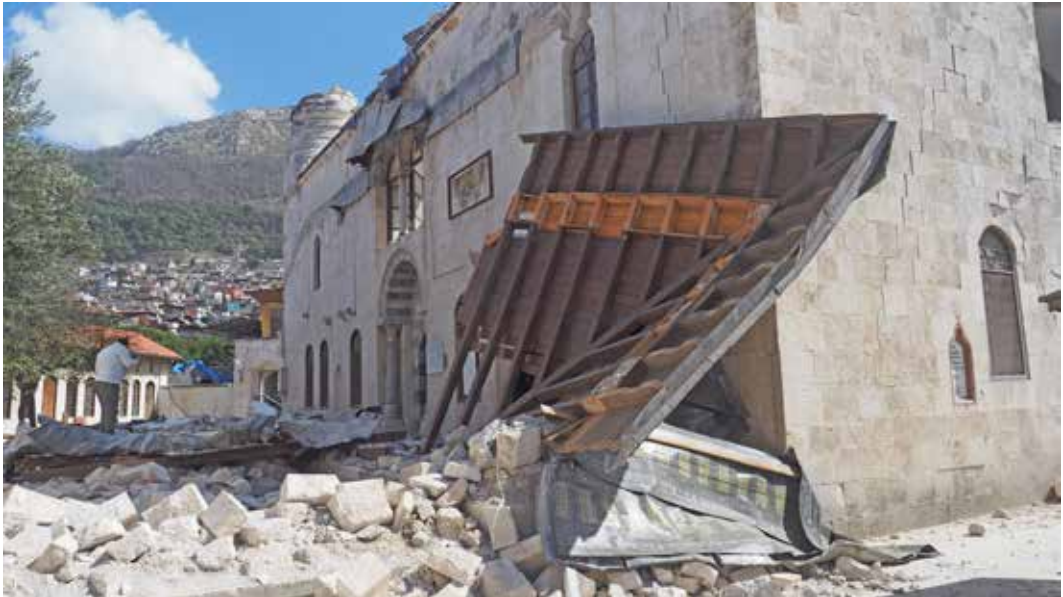
View 1.14 Şeyh Ali Mosque after the earthquake
