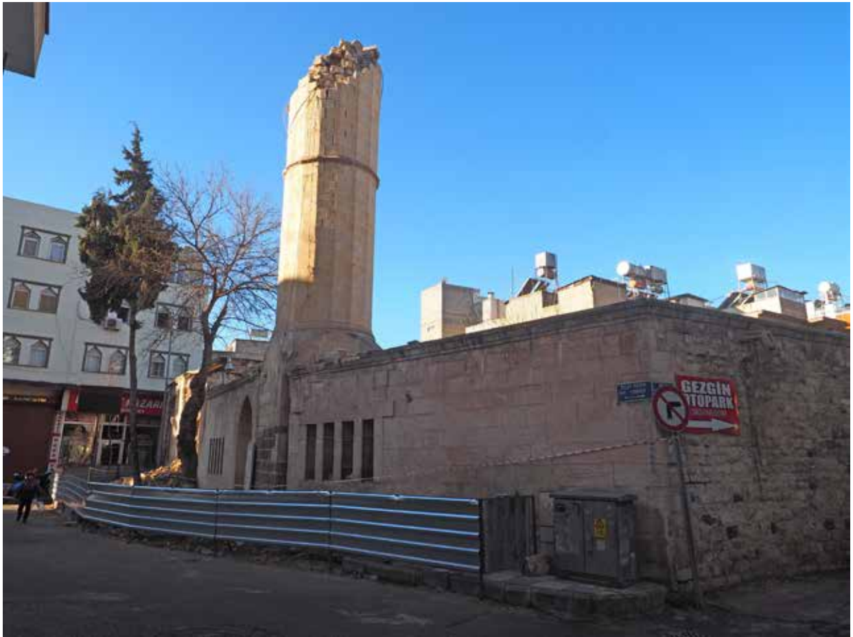
View 2.5 Tabakhane Mosque after the earthquake
