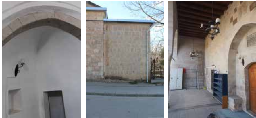
View 7.5 Ak Minaret Mosque after the earthquake
