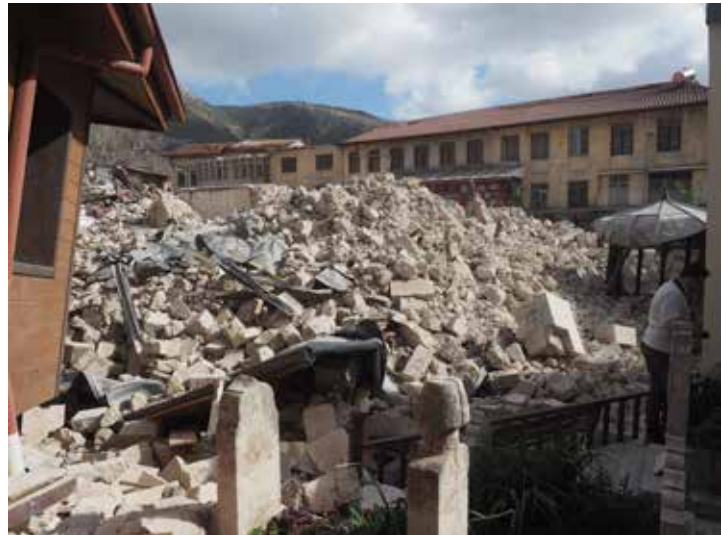
View 1.26 İhsaniye Mosque after the earthquake
