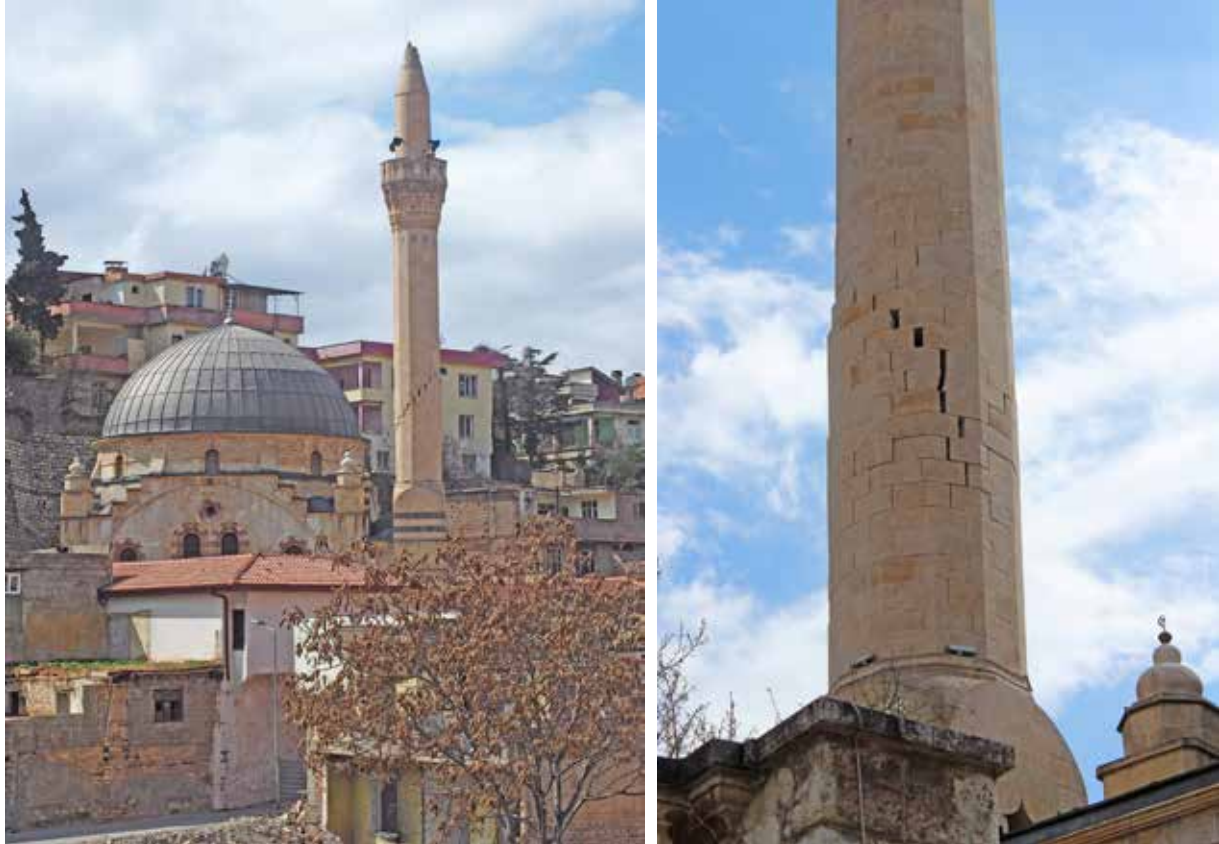
View 8.7 Acemli Mosque after the earthquake
