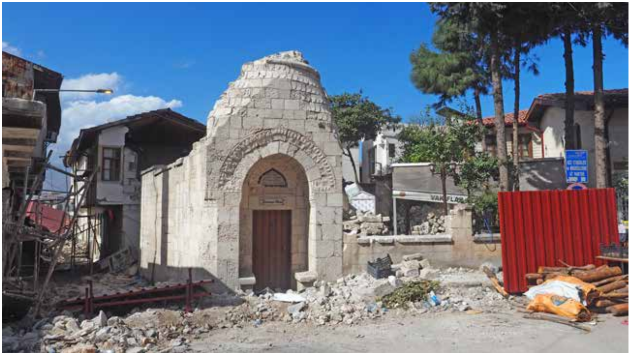
View 1.20 Sarimiye Mosque after the earthquake
