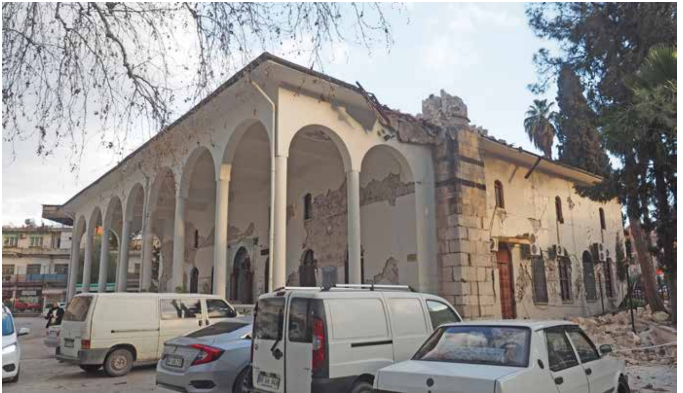
View 9.1 Osmaniyè Envarül Hamit Mosque after the earthquake
