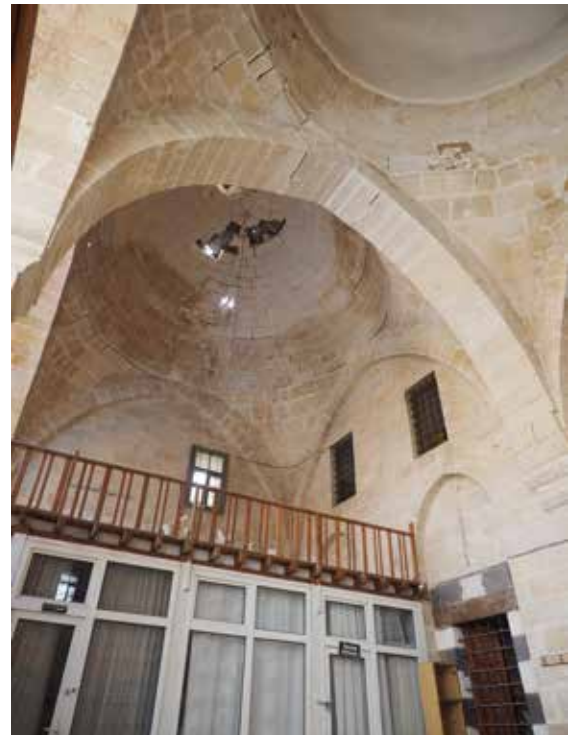
View 3.25 Hüseyin Paşa Mosque after the earthquake
