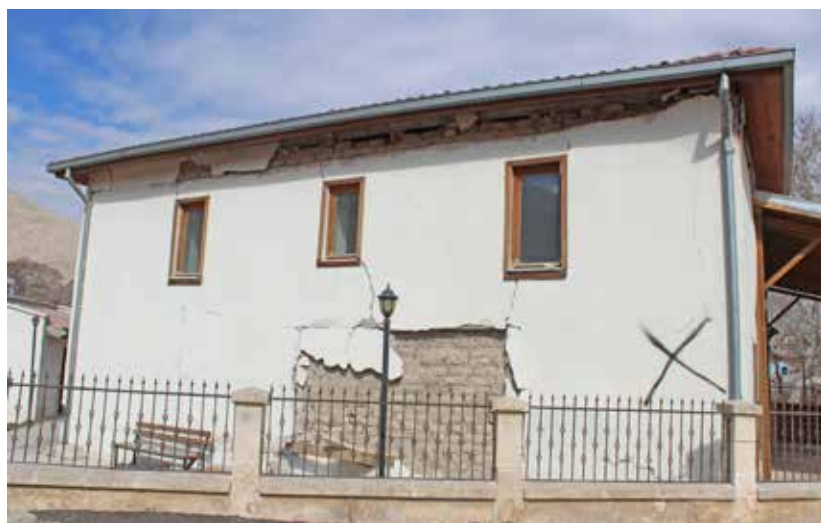
View 8.5 Elbistan Ceyhan Mosque after the earthquake
