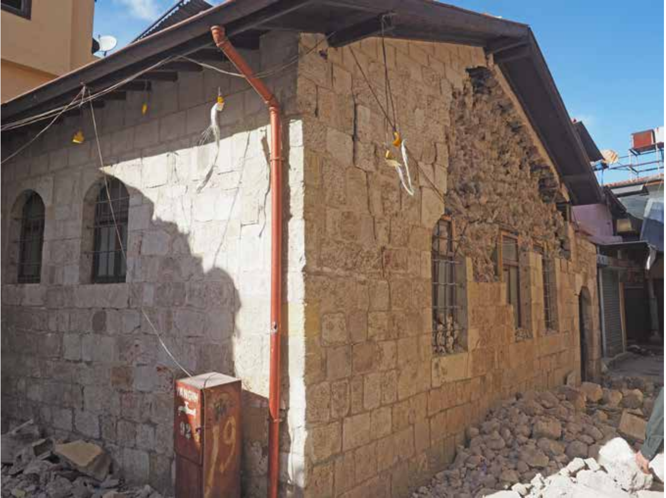
View 1.29 Debruz (Uzun Çarşı) Masjid after the earthquake
