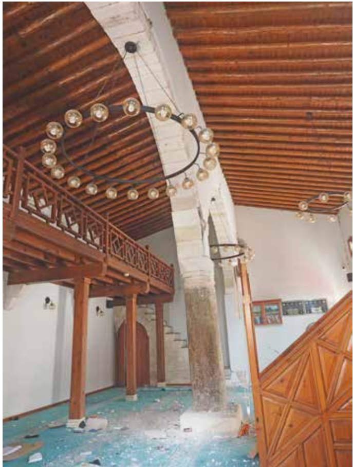
View 1.21 Sarimiye Mosque after the earthquake
