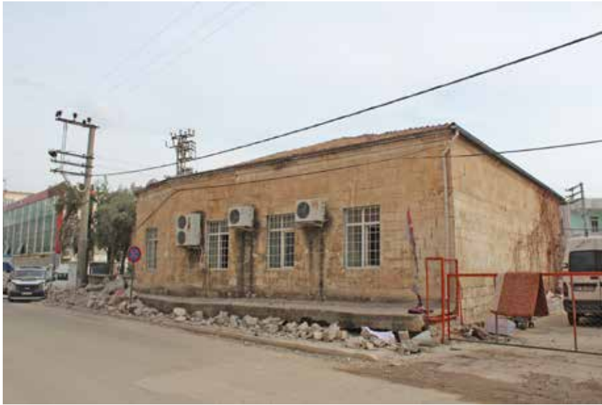
View 5.9 Hacı Süleyman Mosque after the earthquake
