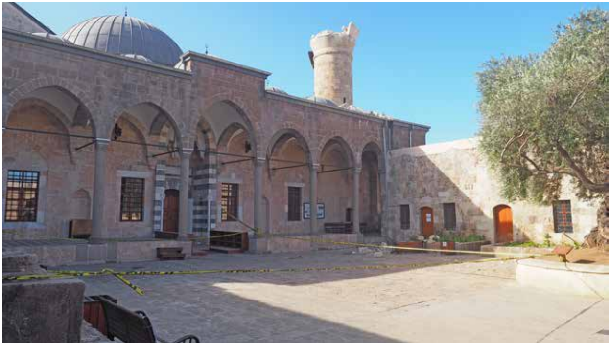
View 1.3 Payas Sokullu Mehmet Paşa Complex after the earthquake
