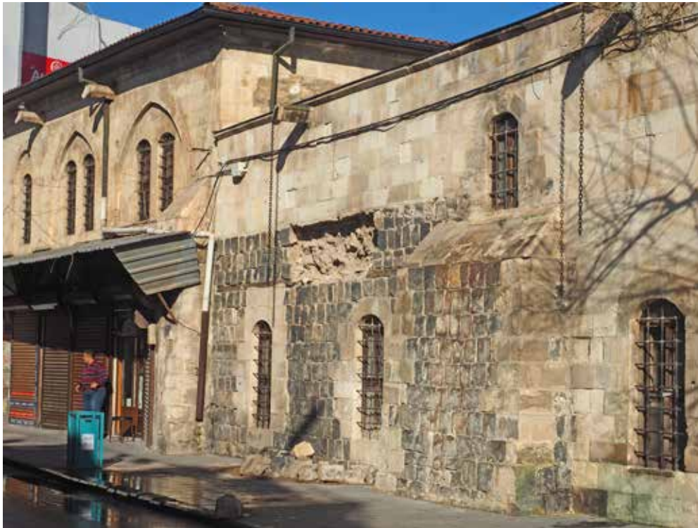
View 2.9 Kara Kadı Mosque after the earthquake
