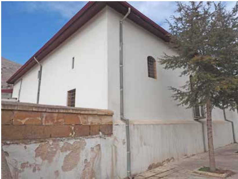
View 8.4 Elbistan Kızılcaoba Mosque after the earthquake
