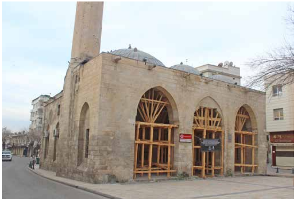
View 4.5 Hüseyin Paşa Mosque after the earthquake
