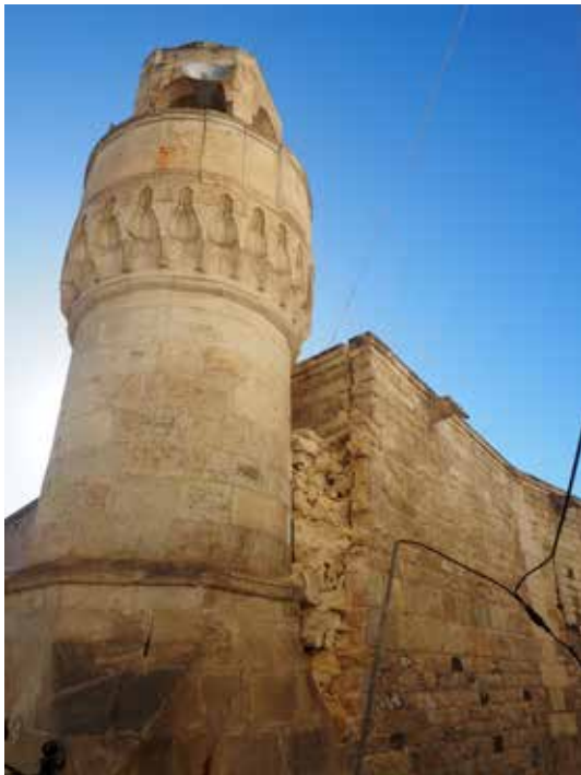
View 2.8 Hacı Derviş Mosque after the earthquake
