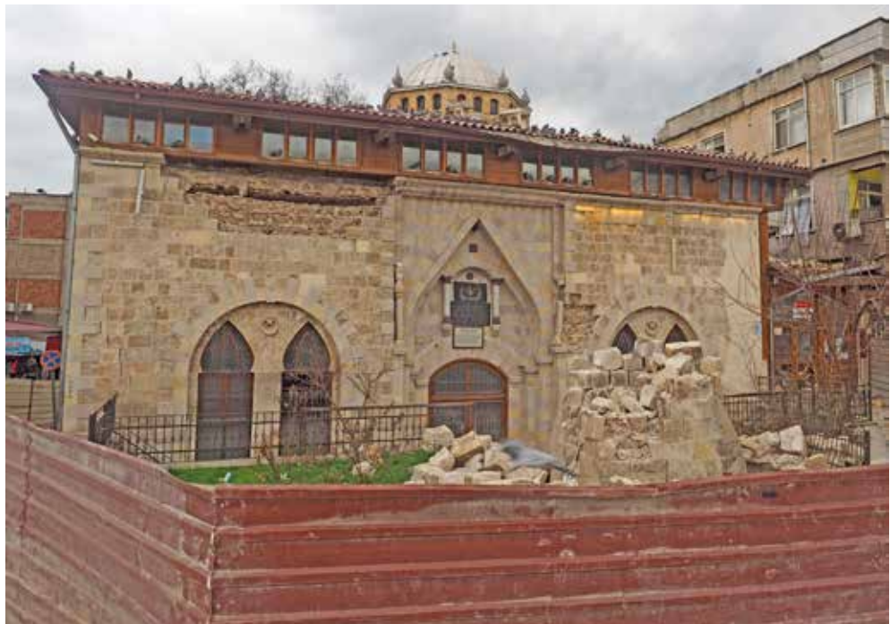
View 8.15 Arasa Mosque after the earthquake
