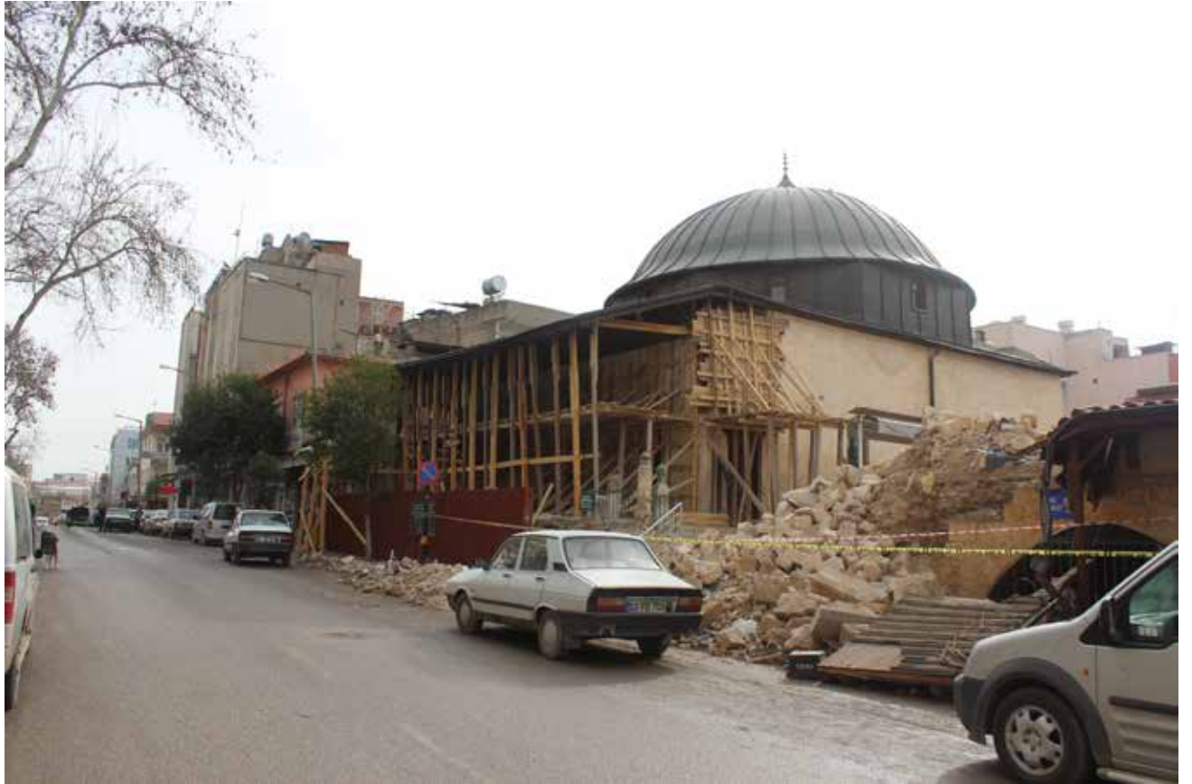
View 5.8 Kab (Hacı Ali) Mosque after the earthquake
