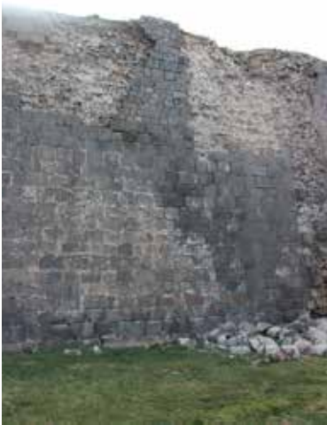
View 6.3 Diyarbakır City Walls after the earthquake
