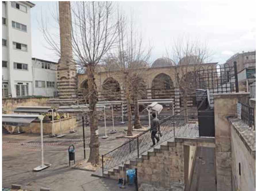
View 3.32 Nuri Mehmet Paşa Mosque after the earthquake
